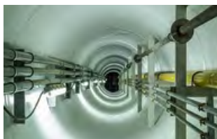
Low pressure pipelines
