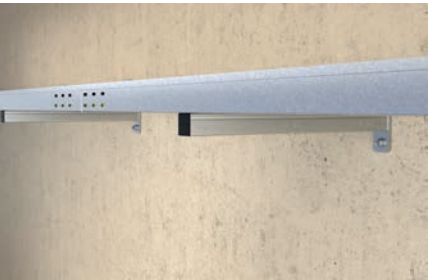
Cable tray on cantilever arm
