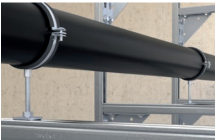
Connection on channel
