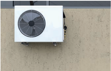
Air conditioner on the outer wall
