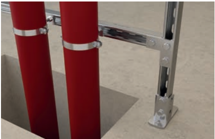
Waste water pipe
