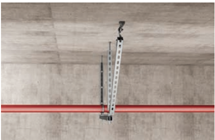
Rod stiffing for vertical seismic support
