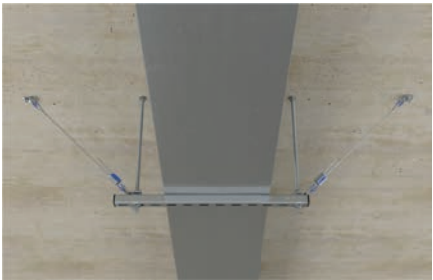
Lateral bracing of ventilation ducts
