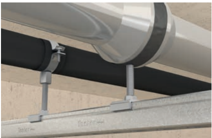
Refrigerant pipe clamps
