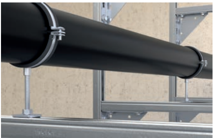
Connection on channel
