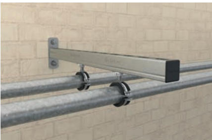
Pipelines on cantilevers
