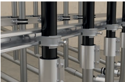
Supply lines fixed to FUS channel
