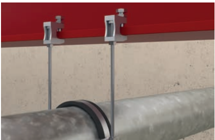
Heavy drainage pipe on beam clamp
