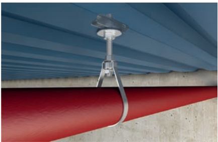
Sprinkler pipe on trapezoidal sheet metal ceiling
