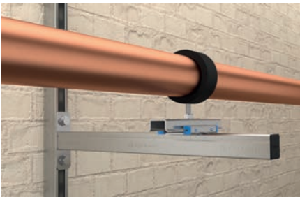
Refrigerant pipe clamp on sliding element
