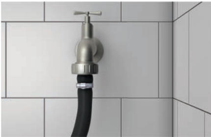
Outlet valve with hose
