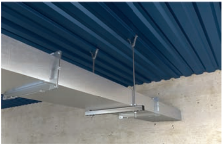
Ventilation duct on trapezoidal sheet
