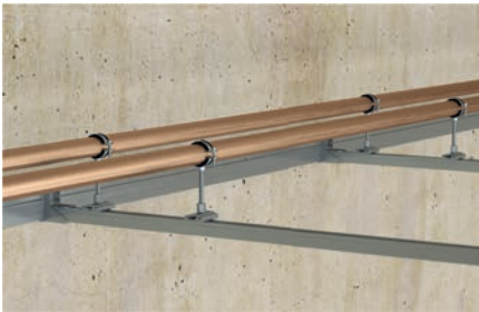
Media lines with thermal expansion
