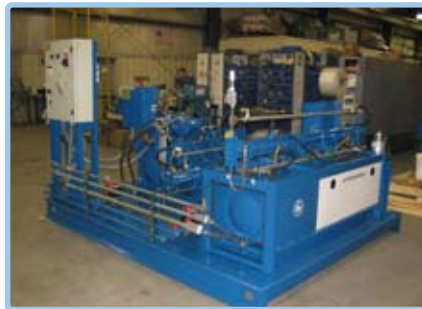
Two compressor package with valve racks and PLC controller.
